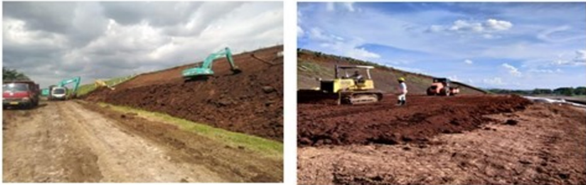
Fig. 7. Excavation of Dam Slope and Embankment of New Material of Lalung Dam Rehabilitation Project.
